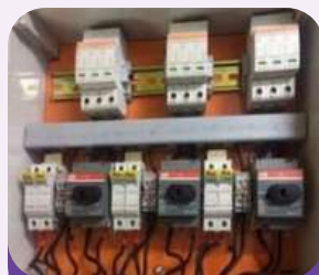
Industrial Junction Box
