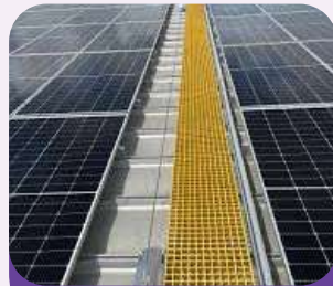
FRP Solar Panel Rooftop Walkway
