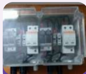
Array Junction Box
