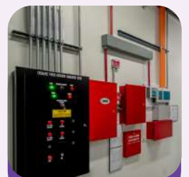
Fire Alarm Cables
